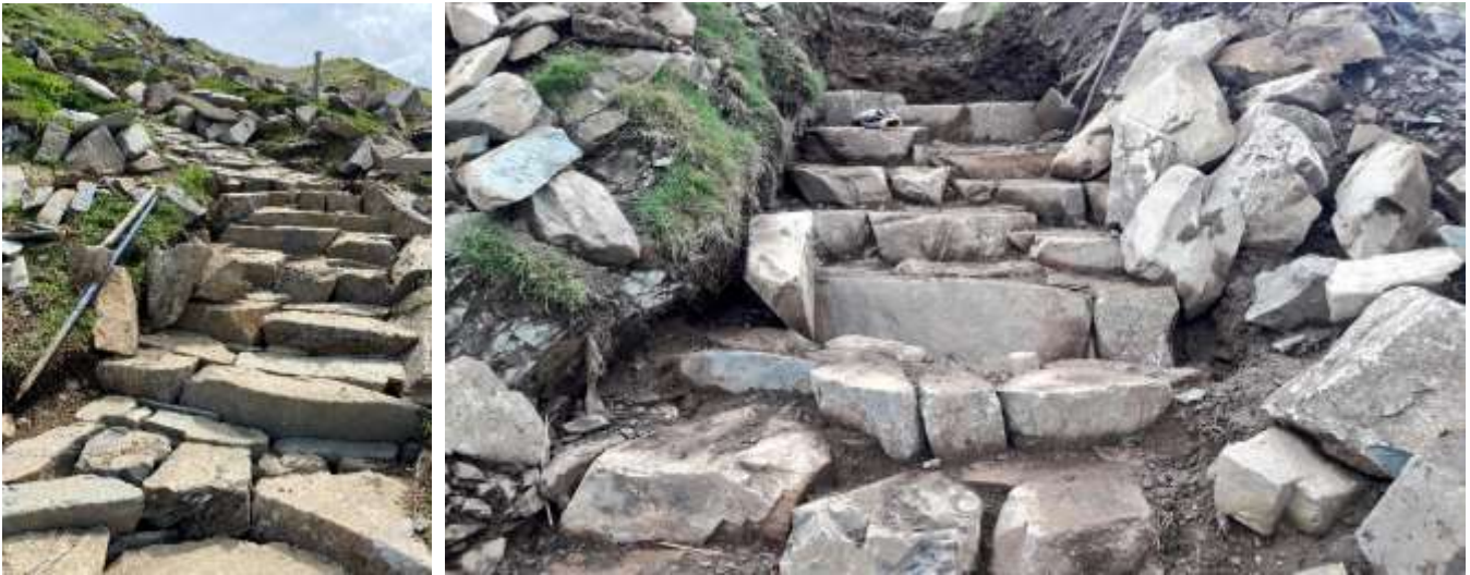
Left - Section of new pitching which has replaced some old sloped stone work. Right - Stone risers through a gully.
