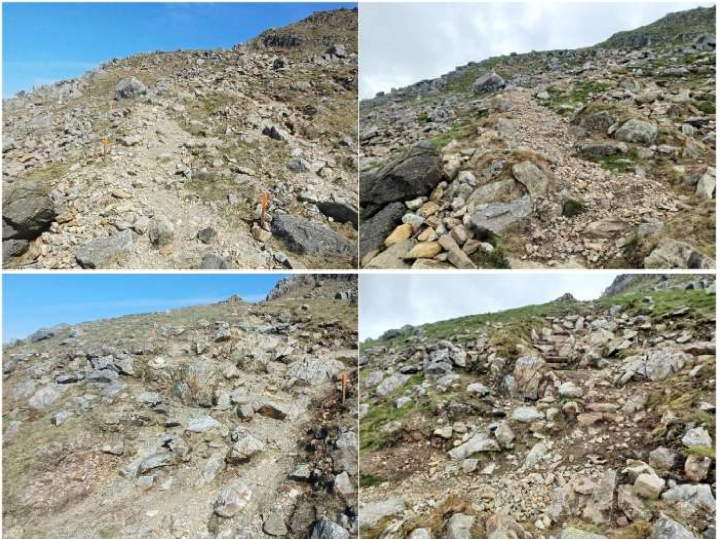
Swirl Hawse before (left) and during (right) work by the South Lakes Ranger team to create a more sustainable path.
