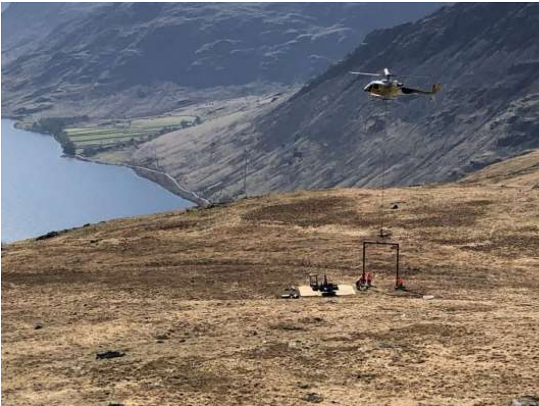
The gantry for rebuilding the digger being flown on to Scafell Pike, Wasdale
