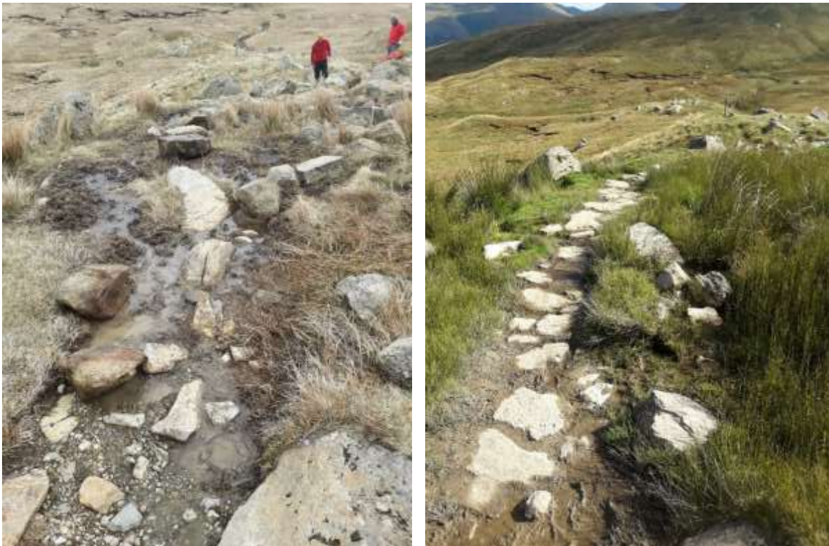
Boggy section of path on Greenup Edge before and after work by the South Lakes team
