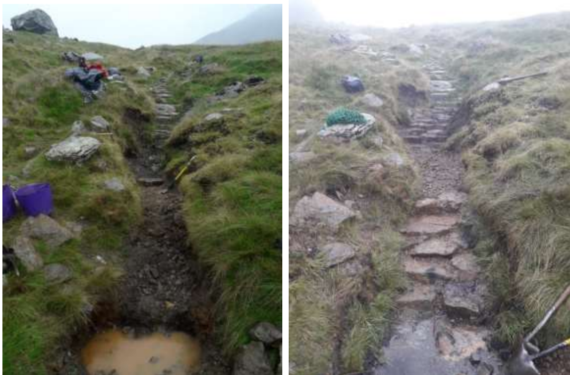
Repairing a badly gullied section of the Coast to Coast at Tongue Ghyll, Grasmere – during (left) and after work (right)
