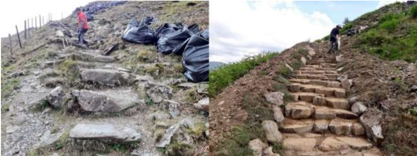
Loughrigg Terrace path before (left) and after (right) removing the old path and installing the new path
