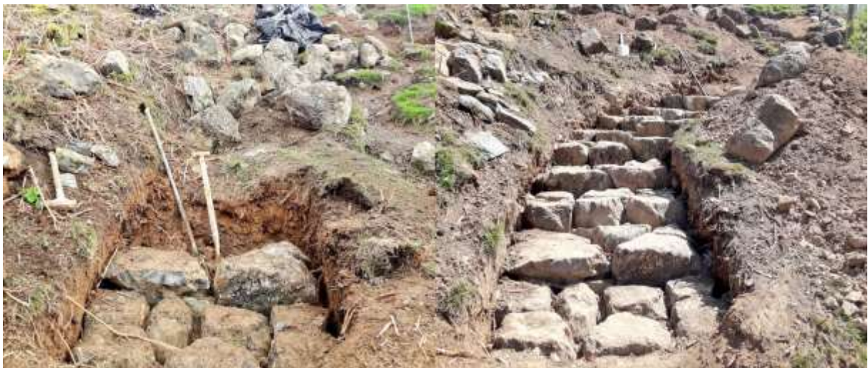
The first courses of pitching on Stone Arthur (left). 10 metre section of pitching on Stone Arthur (right).
