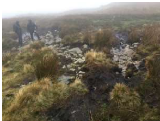
Coast to Coast route over Greenup Edge where a stone-flagged and aggregate path will be created to allow the peatland to heal
