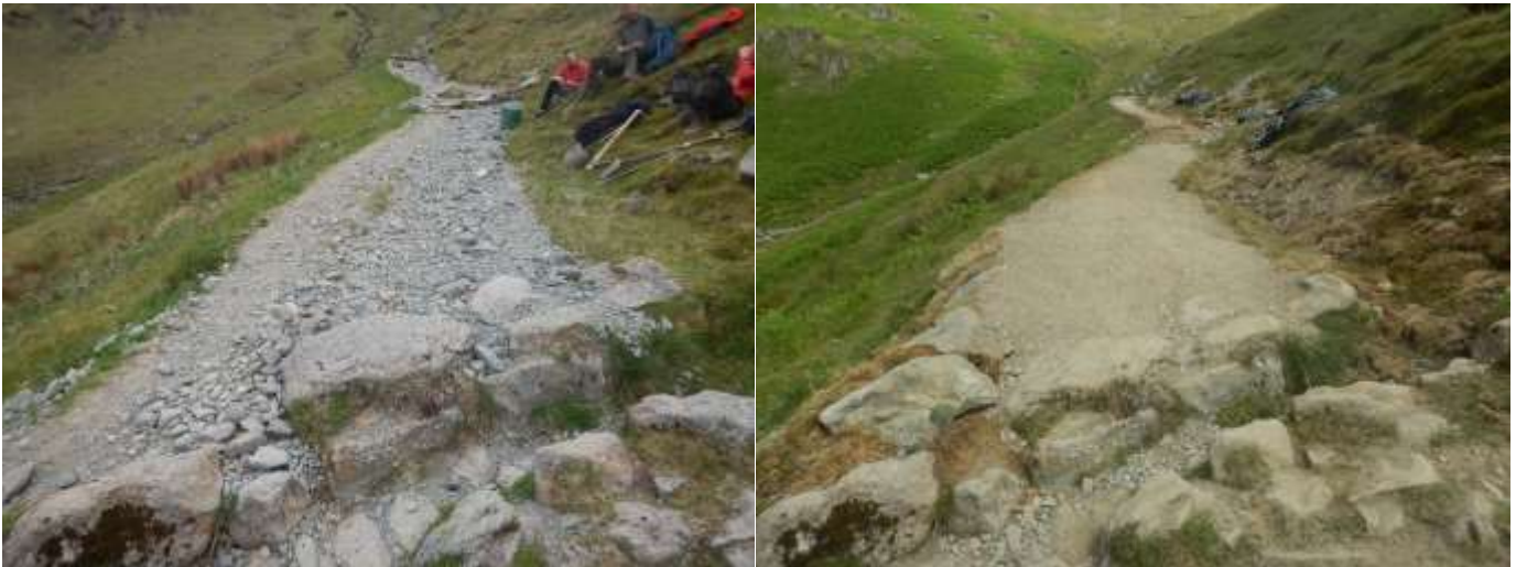
Wythburn path before (left) and after (right) constructing a "roman" style path
