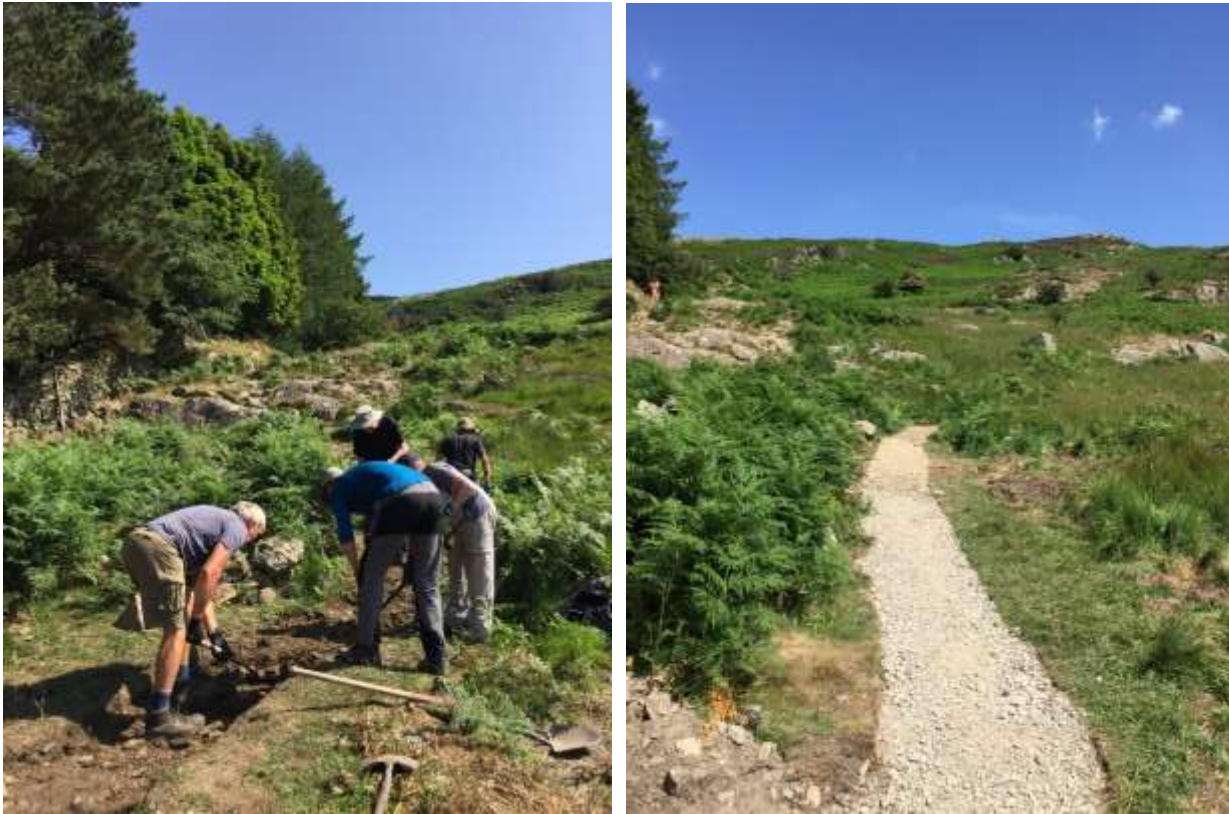
Rangers and volunteers working on the path on Gowbarrow Fell Ullswater (left) and the finished section of path (right)
