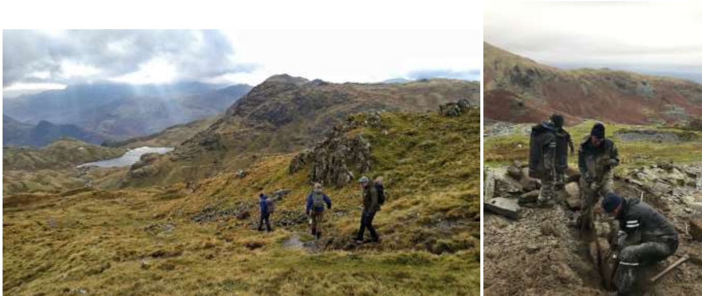
Volunteers descending from Sergeant Man above Stickle Tarn (left) and building a drain on Coniston Old Man (right)
