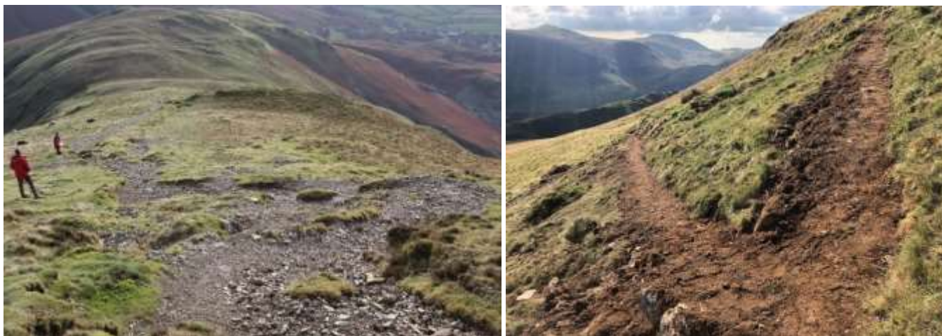
Erosion on Whiteless Pike above Buttermere before work (left) and the newly created bench path (right)
